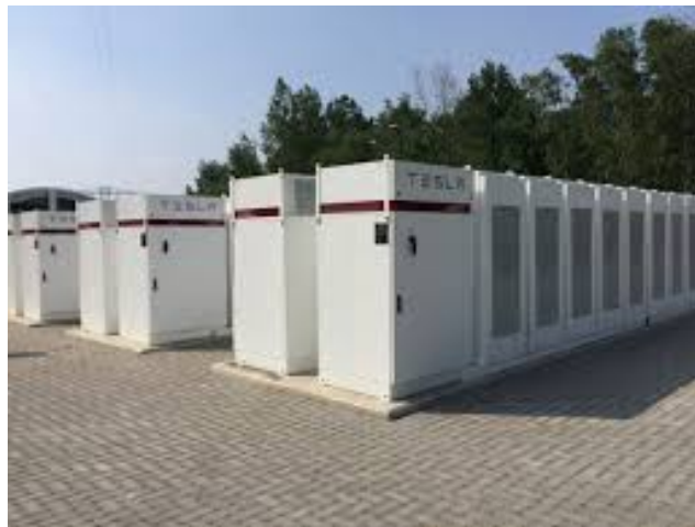
Figure 12 - Tesla utility Scale Storage (source:pv-magazine.com)
