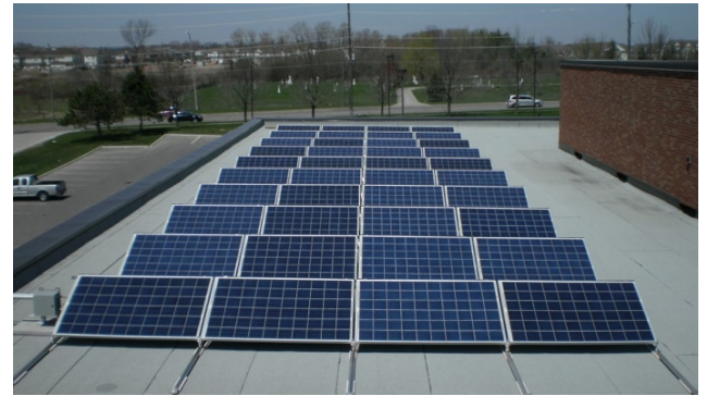
Figure 7 - Typical Roof Mounted Solar System
